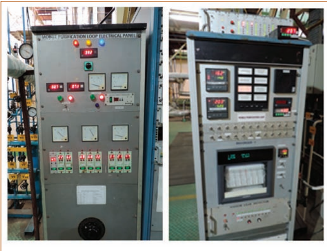
Figure 3: Electrical and instrumentation panels of mobile purification loop
