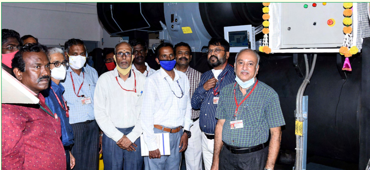
Dr. B. Venkatraman, Distinguished Scientist & Director, IGCAR along with Senior Colleague dedicated during the first 750 TR capacity Centrifugal Chiller at CWCP - II to the centre
