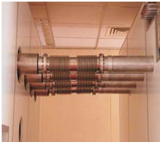
Magnetically Shielded Room Coupled to Radio Frequency Shielded Room via Shielded Waveguides Shielding Factor 70 dB @ 1Hz improving to 100dB @ 100Hz
