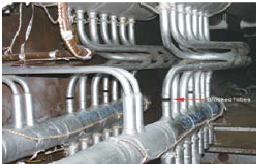
Fig. 1 Modified water sub-headers
