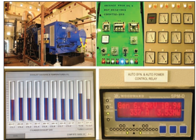
Fig. 5 Diesel generators in place
