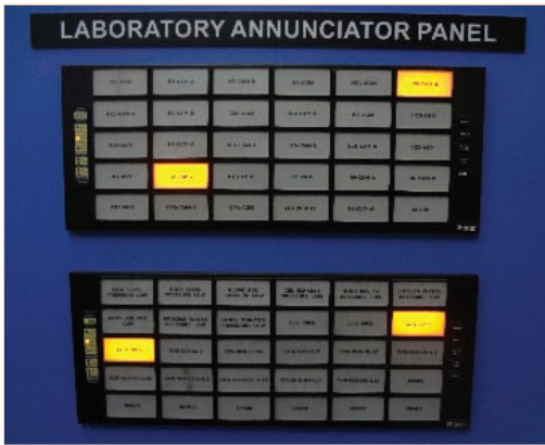
Fig. 2 Photograph of annunciator panel
