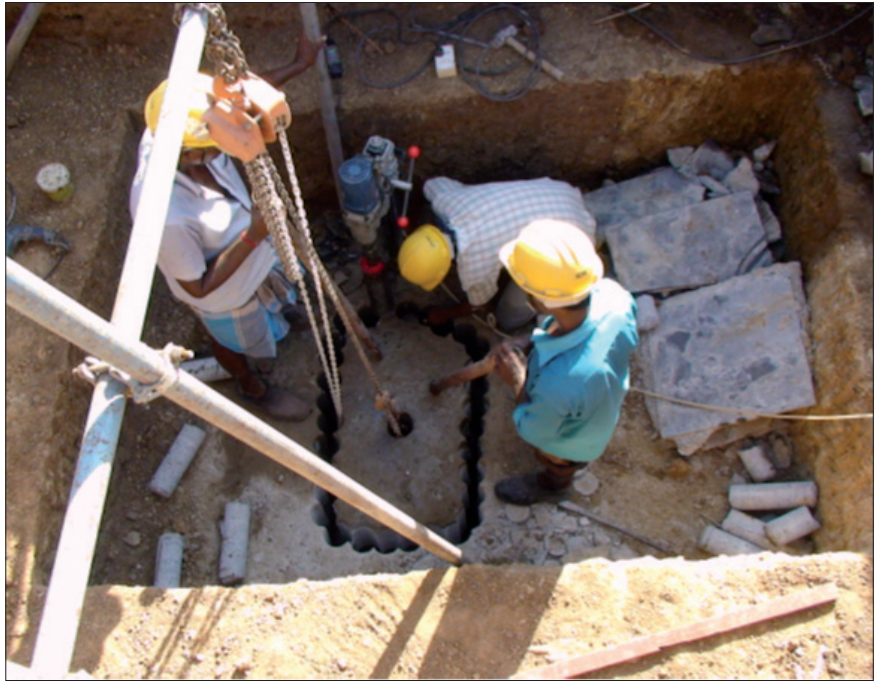
Fig. 1 Core cutting the top cover slab with drum type diamond core cutter
