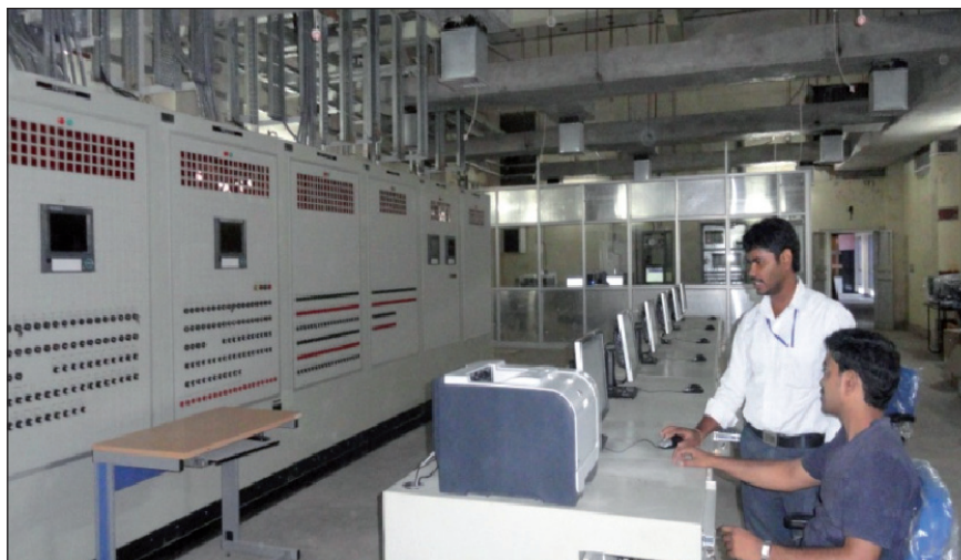
Fig. 2 Main control panel and consoles of DFRP
