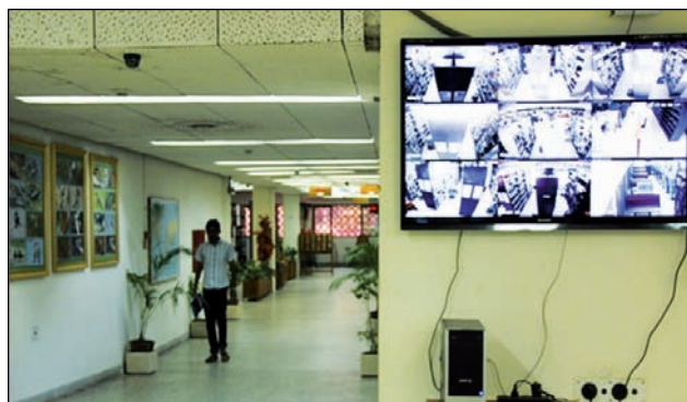
Fig. 2 CCTV display at SIRD
