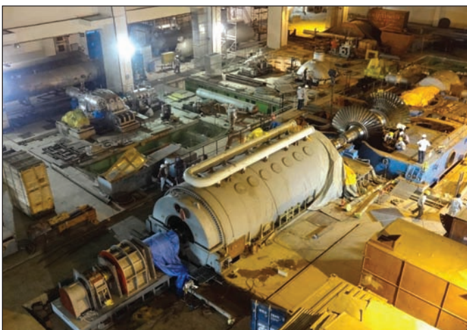
Fig. 6 Overall view of turbine floor
