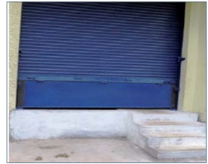
Fig. 4 Rolling shutters with leak tight flood barriers
