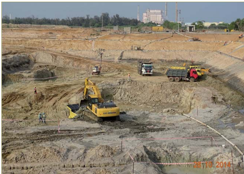
Fig. 1 Excavation activity on trial pit in plant area of FRFCF in progress
