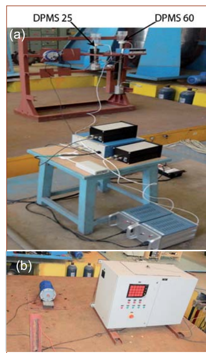
Fig. 2 Test arrangement for the (a) differential pressure monitoring system and (b) material airlock control panel
