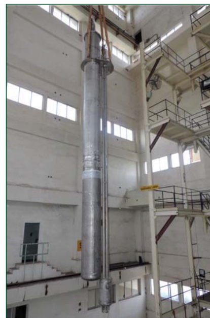
Fig. 3 Erection of integrated cold trap in test vessel-3 of large component test rig sodium loop
