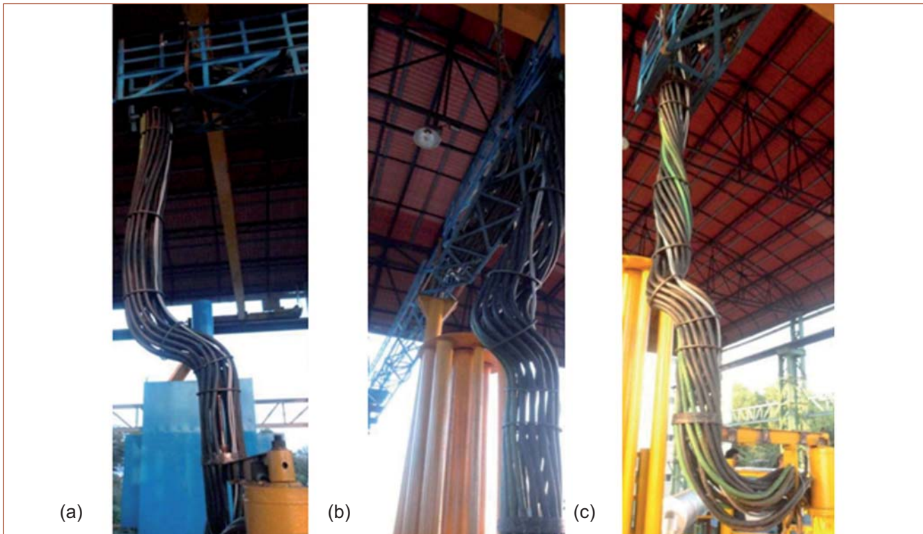
Fig. 5 Profile of trailing cables under different plug positions (a) SRP-0° & LRP-0°, (b) SRP-0° & LRP-360° and (c) SRP-180° & LRP-360°
