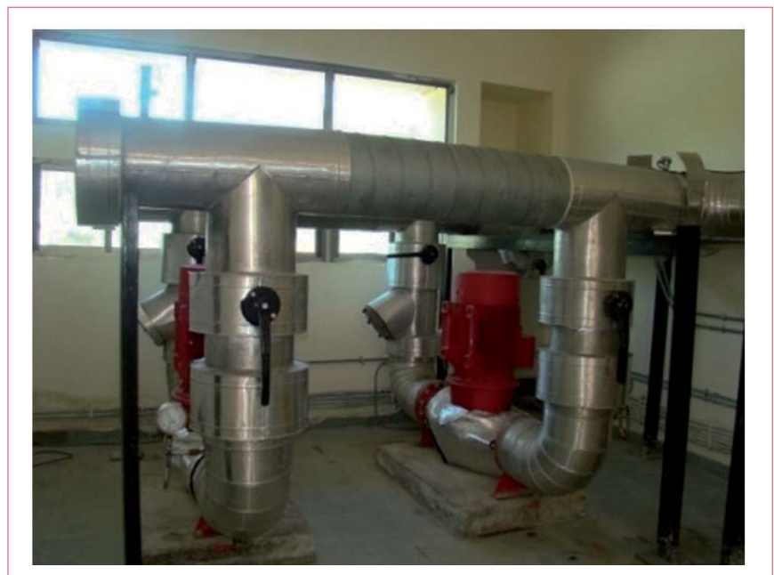
Fig. 2 Chilled water pump installation
