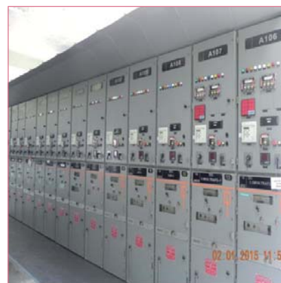
Fig. 1 Bus section along with the bus duct
