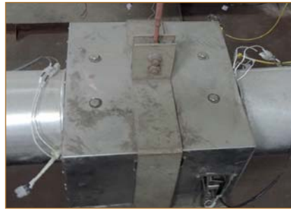
Fig. 1 Flowmeter in dump line
