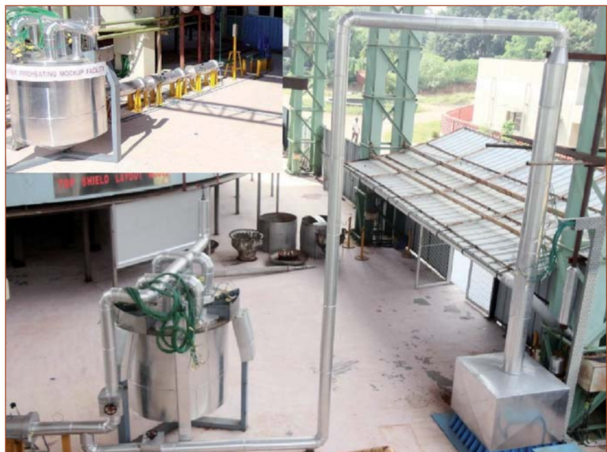
Fig. 2 Reactor assembly and fuel subassembly mock-up facilities
