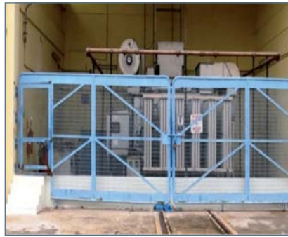
Fig. 3 Outdoor transformer cubicles provided with short brick walls
