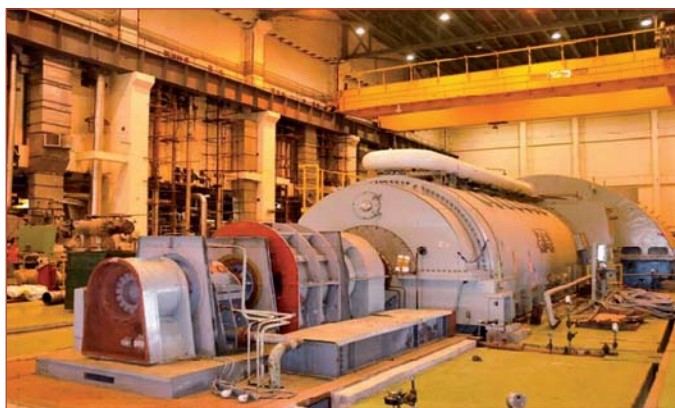
Fig. 3 Overall view of turbine floor
