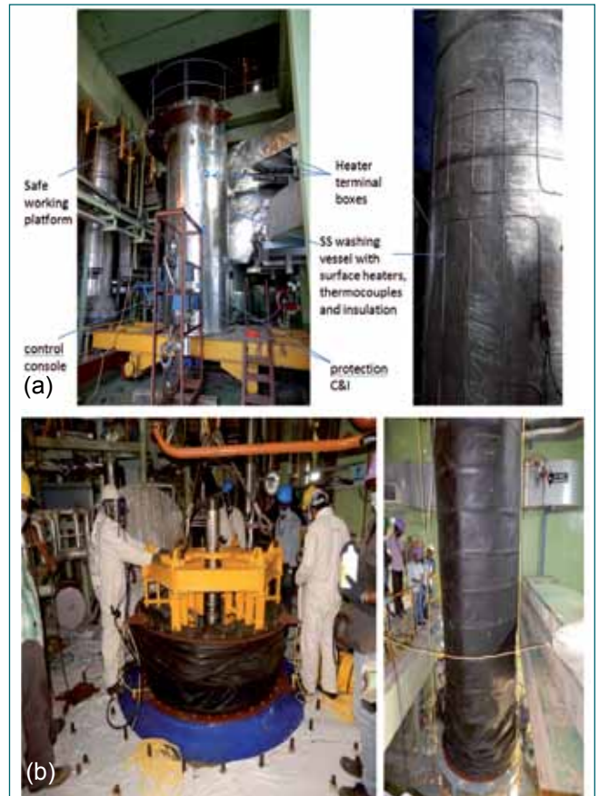
Fig. 2 (a) Na washing facility including control console & protection C&I and (b) retraction of pump internal assembly of SSP-2
