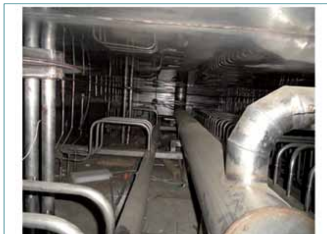
Fig. 2 View of limited head room space 600 mm between top surface of the containment box and concrete wall
