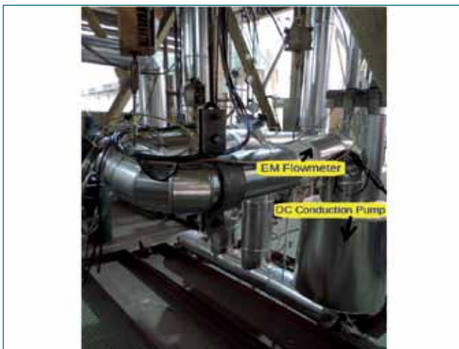
Fig. 4 Photograph of DCCP in test loop
