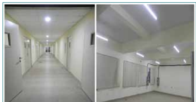
Fig. 2 Corridor and laboratory at MMG II illuminated by 48V LED fixtures
