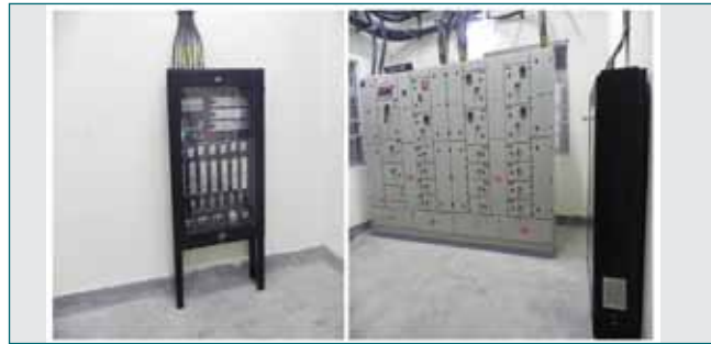
Fig. 1 Converter panel in electrical room
