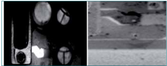
Fig. 2 Thermography images of failed location
