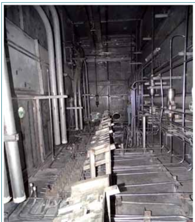
Fig. 1 Typical inside view of containment box with equipments and piping
