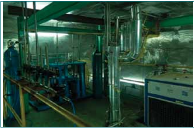
Fig. 4 RISHI Loop with MI level probe
