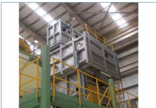
Fig. 1 Hood installed over the containment box
