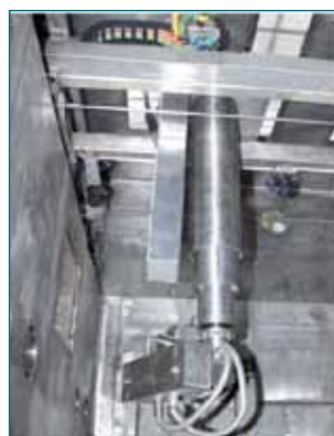
Fig. 1 Power manipulator in operation inside CB
