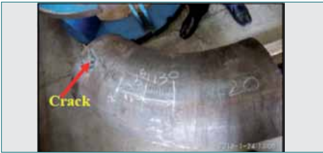
Fig. 3 Crack at 40° bend angle
