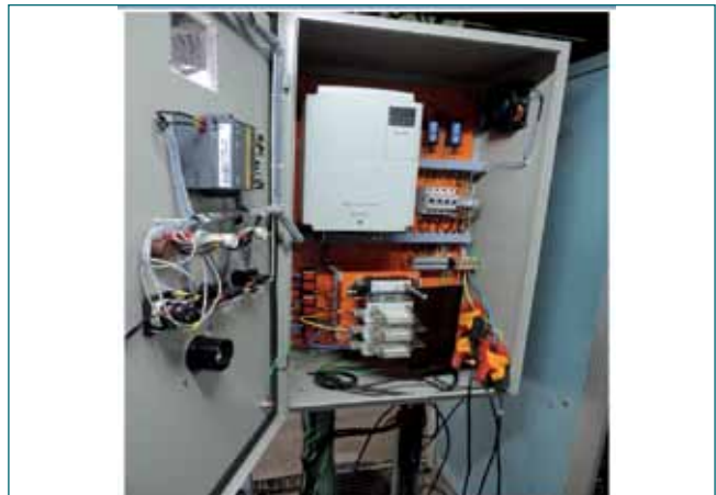
Fig. 2 Photograph of variable frequency drive
