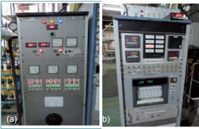
Fig. 3 (a) Electrical and (b) instrumentation panel of mobile purification loop
