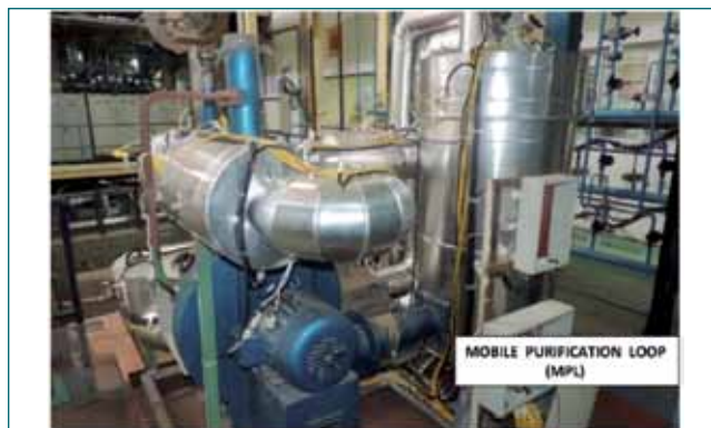
Fig. 2 Re-commissioned mobile purification loop
