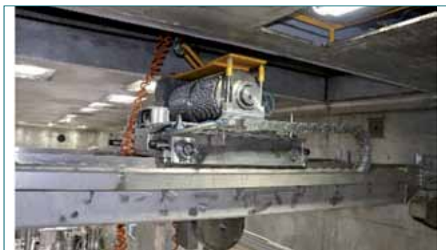
Fig. 2 Two ton hoist installed inside the hood
