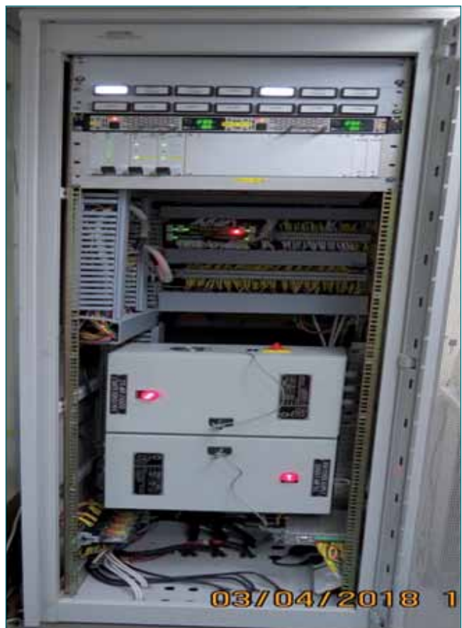
Fig. 2 Drive electronics installed in panel
