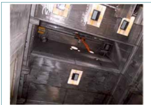
Fig. 3 Hoist viewed from bottom of hood
