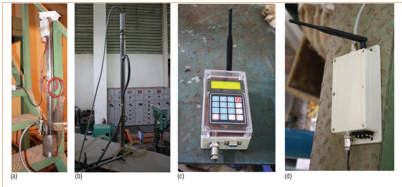
Figure 4: Level measurement system (a) DP Sensor, (b) probe inserted to tank, (c) wireless receiver and (d) wireless transmitter
