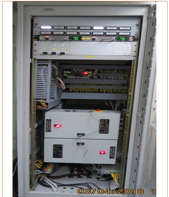
Figure 2: Drive Electronics installed in panel
