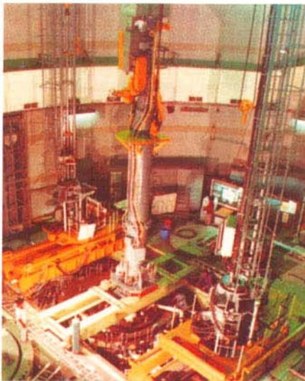
Towering high - Special Flast-2 on the Reactor flanked by Charging and Discharging Flasks
