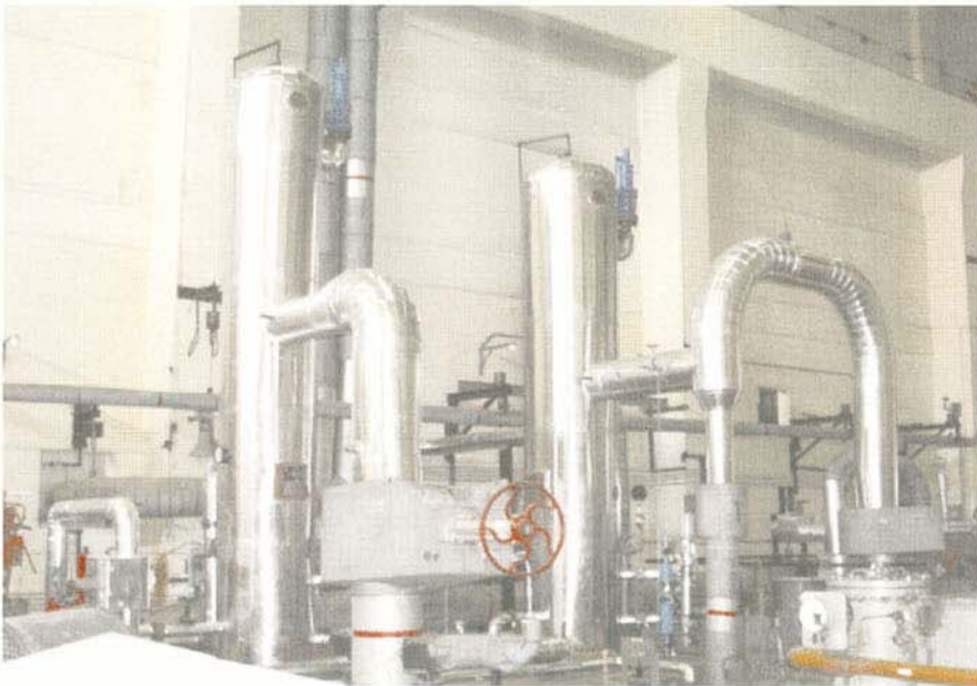
Fig. 3 : Low Pressure Heaters # 1&2
