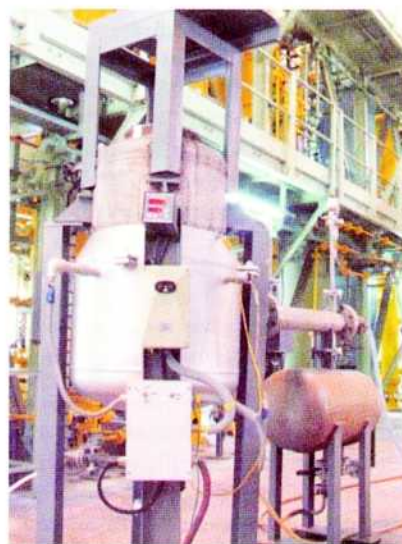
Fig.2 A view of evaporator used for evaporating enriched boric acid solutions
