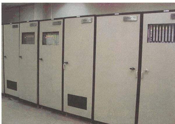
Modern safety critical Real Time Computer System for FBTR
