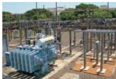
Central Switching Station
