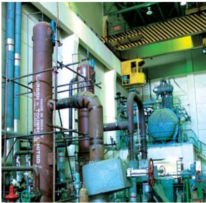
Fig. 4. Shell and Tube type reheaters
