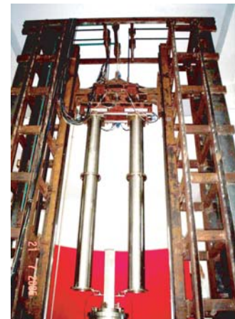
Fig. 1. Poolside spent sub-assembly inspection bench
