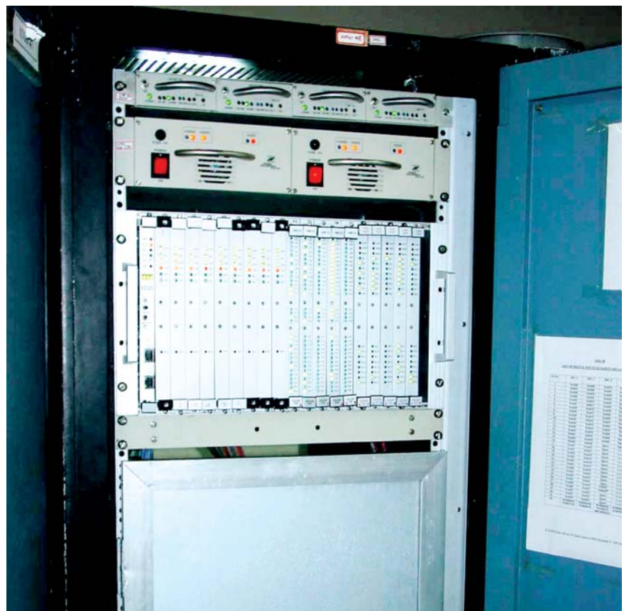
Fig. 1. New Central Data Processing System of FBTR
