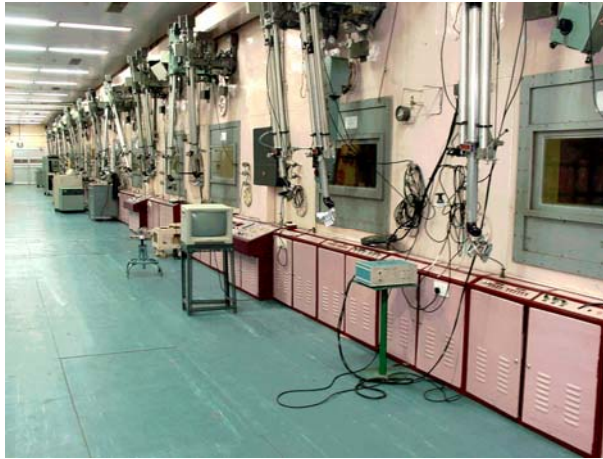
A view of the operating area of Hot cells
