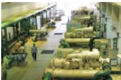
Array of compressors to "chill" the water
