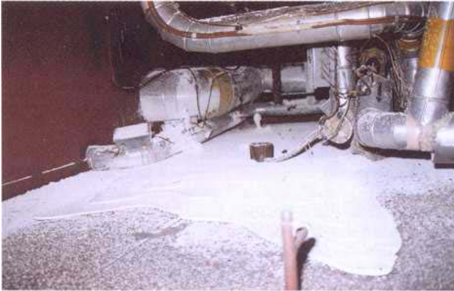
Fig. 1 : Floor of the purification cabin covered with leaked sodium.
