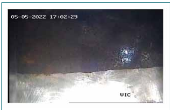
Fig.3: Dissimilar weld seen by visual inspection camera (VIC)
