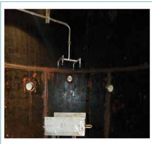
Fig.1: Combustion chamber with multi-nozzle injection system and disposal tray
