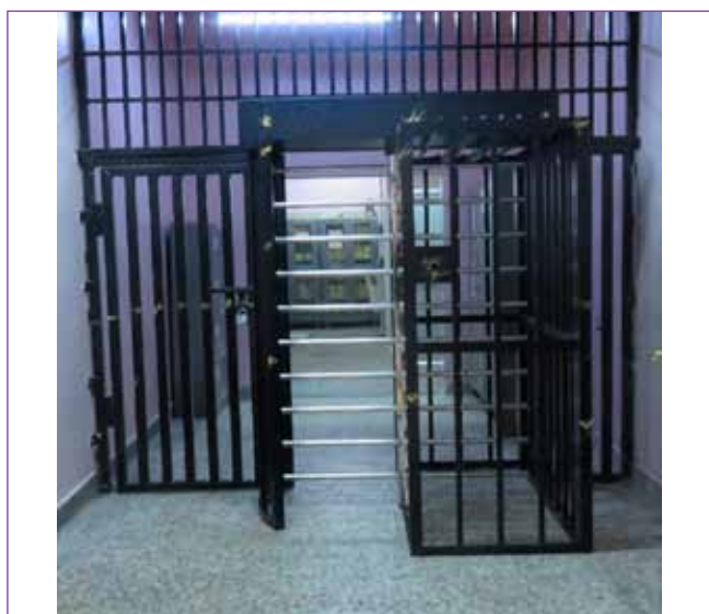
Fig.1: One way entry through turnstile gate to active areas of FBTR
