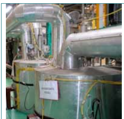
Fig. 2: Salt storage vessel with transfer line
