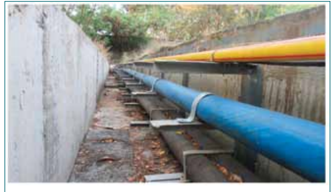
Fig. 3: 33kV cable from NCSS-3 to CSS in trench
