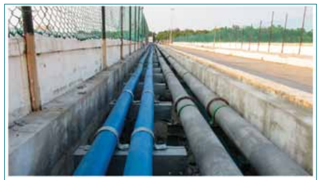
Fig. 4: 33kV Cable over Edaiyur Bridge
