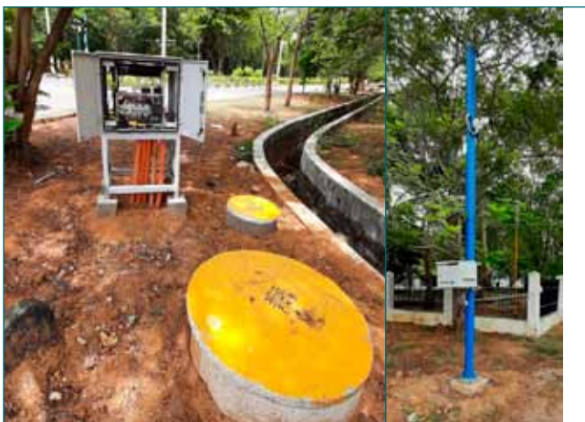
Fig.1: View of Junction box MHC Earth pit and pole in the field
