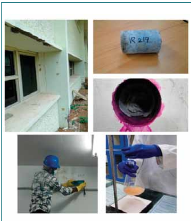
Fig. 1: Damaged RC column and condition survey
