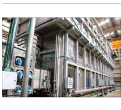
Fig. 1: PPRDF 500 m^3 Containment Box
