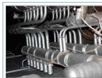
Fig. 9: Inlet water sub-header welded to FBTR SG module
