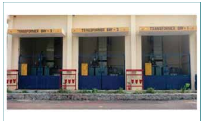
Fig. 3: 2 MVA transformers of 11/0.415kV Oil type
