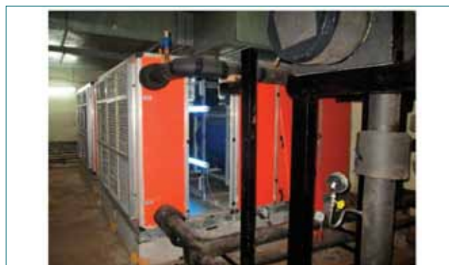
Fig. 3: AHUs revamped at HASL building
