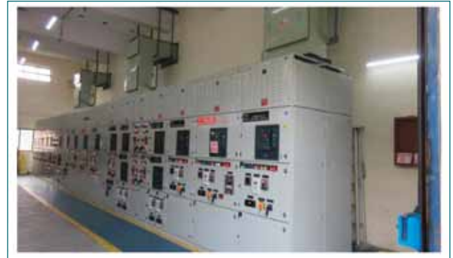
Fig. 2: LT Switch board with Bus-duct at PDC XI substation
