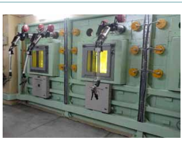
Fig. 2: TDFRP Contactor cell lighting arrangement
