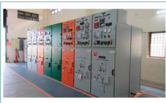
Fig. 1: 11kV Switch board at PDC XI substation
