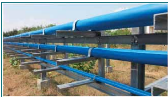
Fig. 2: OFC cable and 33kV Cable 2 runs from NCSS-2 to NCSS-3 and cable between NCSS-3 and CSS
