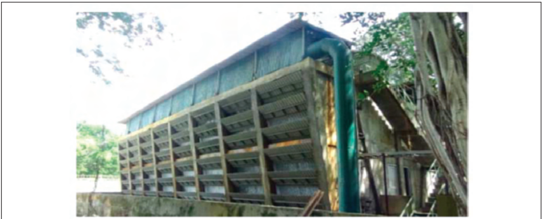
FBTR cooling tower
