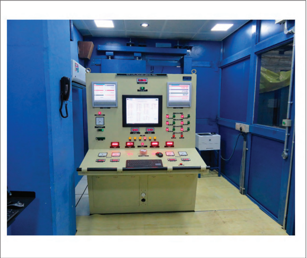
Supplementary control Room
