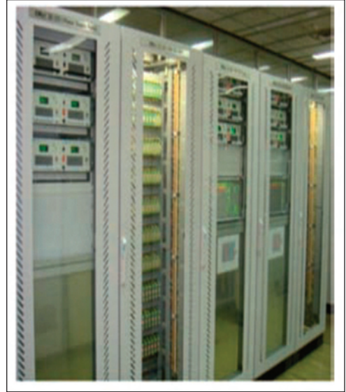
Fault tolerant Real time computer systems of FBTR
