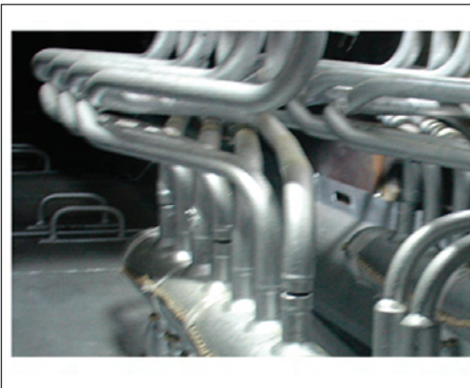
Tubes of SG in blanked condition
