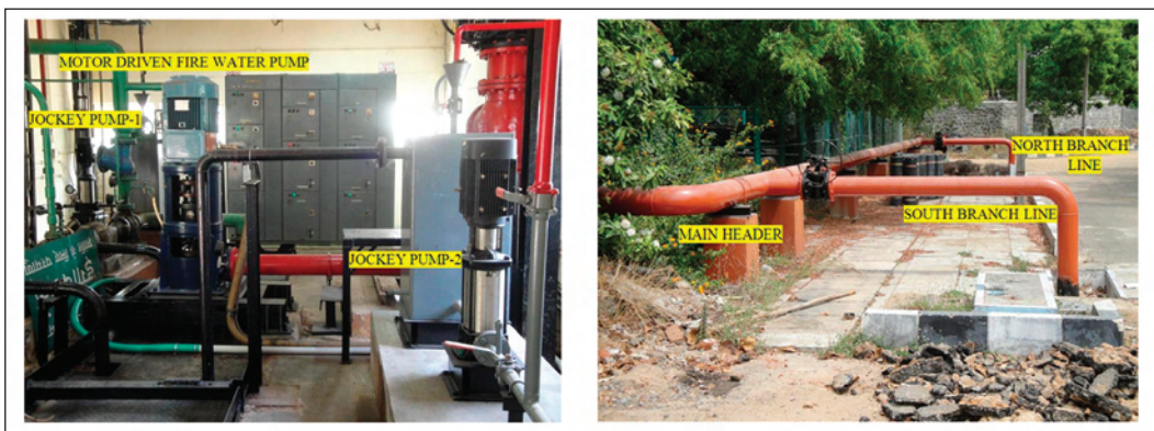
Motor Driven water system
