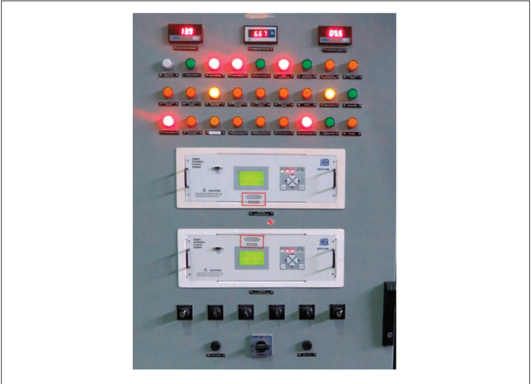
AVR Controls in Control Room
